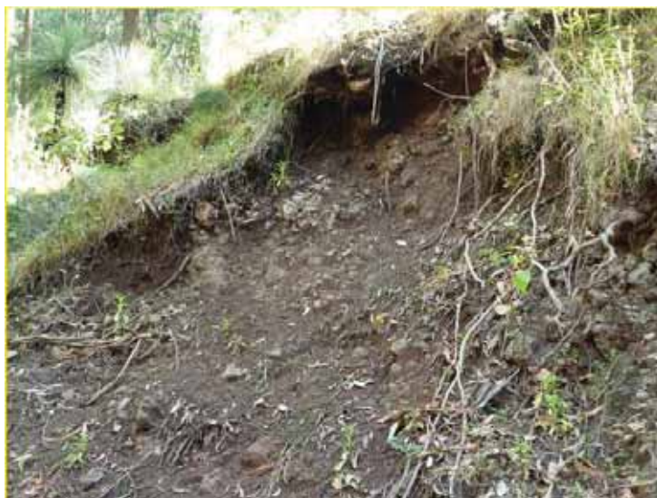
Figure 3.11 Soil creep and possibly recent soil loss at Cascades Trail road cutting
