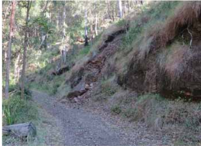
Figure 3.7 Rockfall in general Project area
