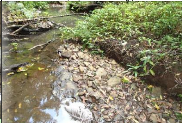
Photo 3.4 Recent erosion on a vegetated sidebar immediately downstream of the proposed crossing.
